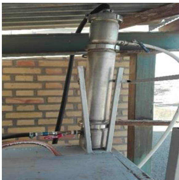
Figure 2. Water scrubber tower
