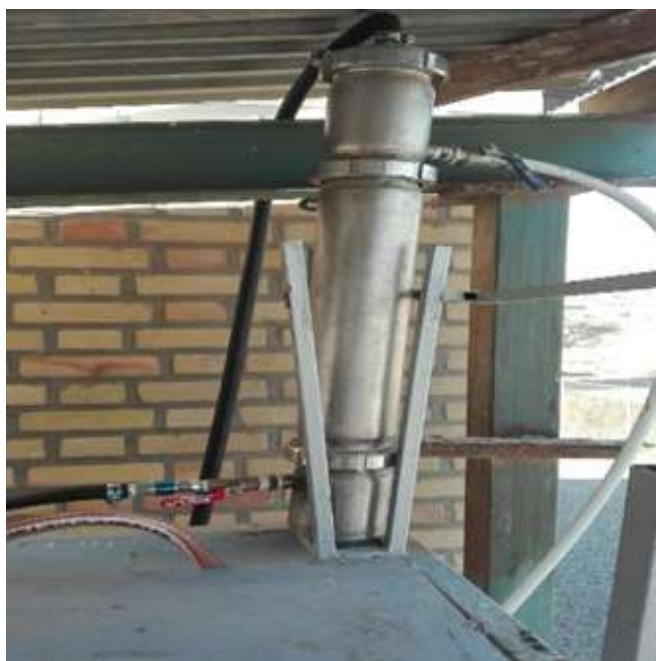
Figure 2. Water scrubber tower
